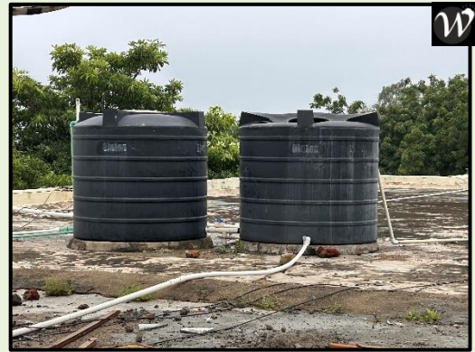
Figure 2. Water tank system in college
