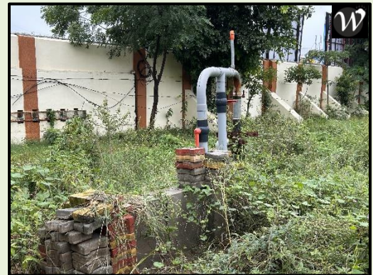
Figure 3. Bore well system in college campus
